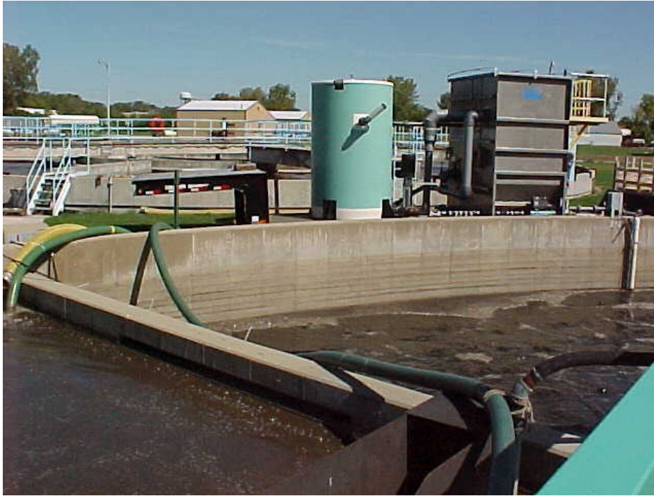
Figure 2: AquaDisk® Test Unit at South Beloit Water Pollution Control Facility
