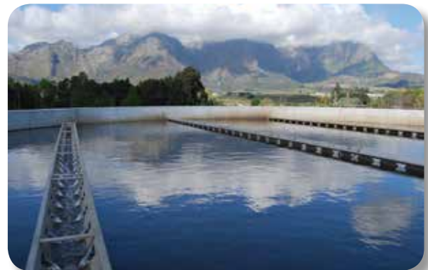
Treated effluent produced from an AquaNereda® reactor.
