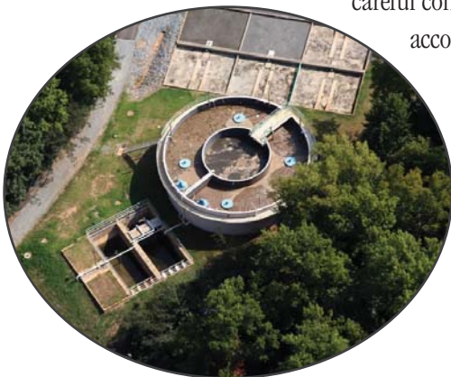
Overview of Warm Spring WWTP's AquaSBR ® system with integral digester in the center.
