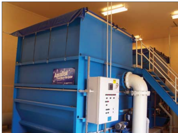
The two AquaDisk ® filters are housed inside a building.
