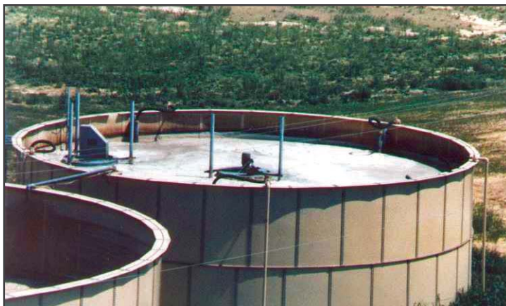
Single basin AquaSBR ® system measures 47' in diameter x 16' SWD.
