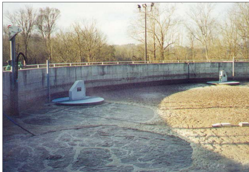
One of the two AquaSBR ® basins during the React Phase of treatment.
