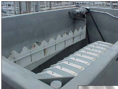
Orange County's North Plant AquaDisk® Filters utilize pile cloth media.
