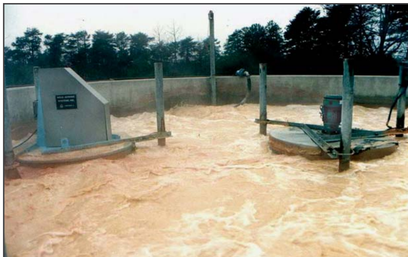
One of the AquaSBR ® basins in operation.
