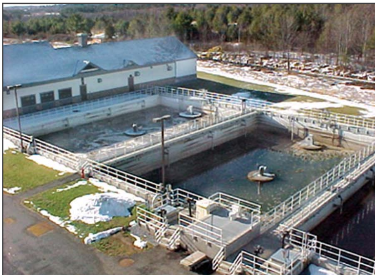
Two of the four AquaSBR ® basins at Middlebury WWTP.
