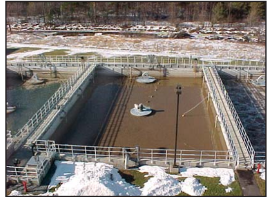
Each of the four basins at Middlebury WWTP measures 82'x55' with an 11.2' LWL and an 18.0' HWL.
