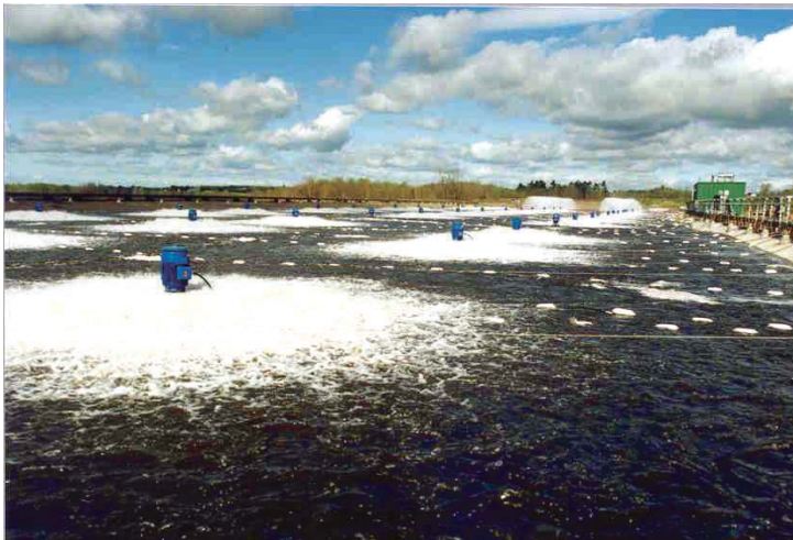
A number of MacLaren's Aqua-Jet ® aerators in operation. Also shown toward the back are the ThermoFlo ® spray coolers in an adjacent basin.
