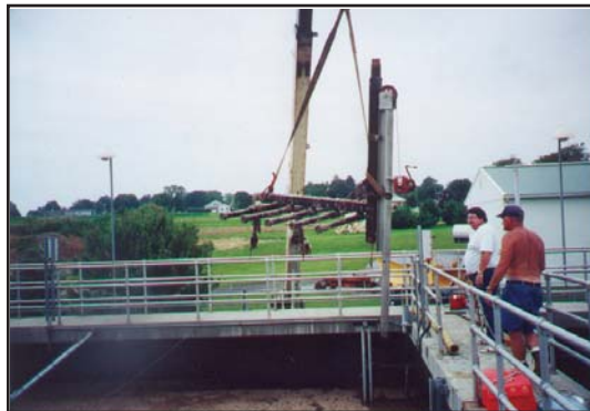
One of the old retrievable coarse-bubble diffuser racks being removed from the basin.
