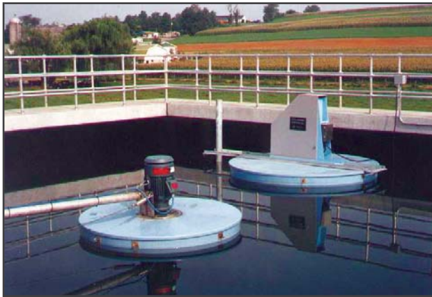
One of the AquaSBR® basins at Leacock Township.
