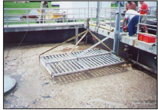
The new fine-bubble assembly on the existing track is being lowered into the basin.
