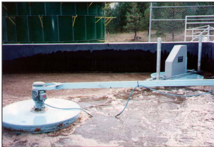
One of the basins containing AquaSBR ® system equipment.
