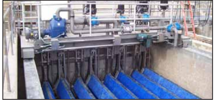
Figure 4 - Existing Traveling Bridge Sand Filter Converted to Cloth Media Diamond Filter
