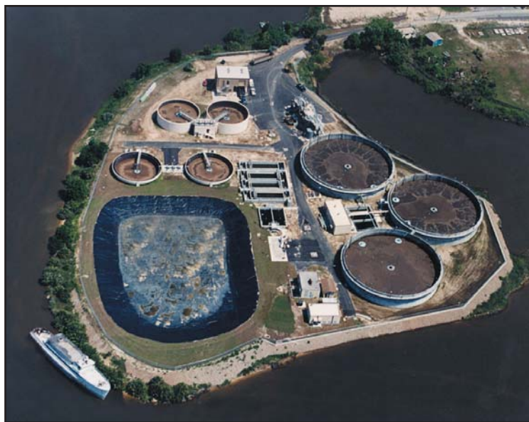
Millville's 3-basin AquaSBR ® system is shown on the right and (4) AquaABF ® sand filters are shown adjacent to the post aeration basins.
