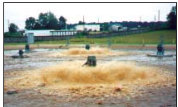
One of the AquaSBR basins in operation at Birds Eye Foods. Shown are the Aqua-Jet aerators in operation and a couple of the AquaDDM mixers are to the left.
