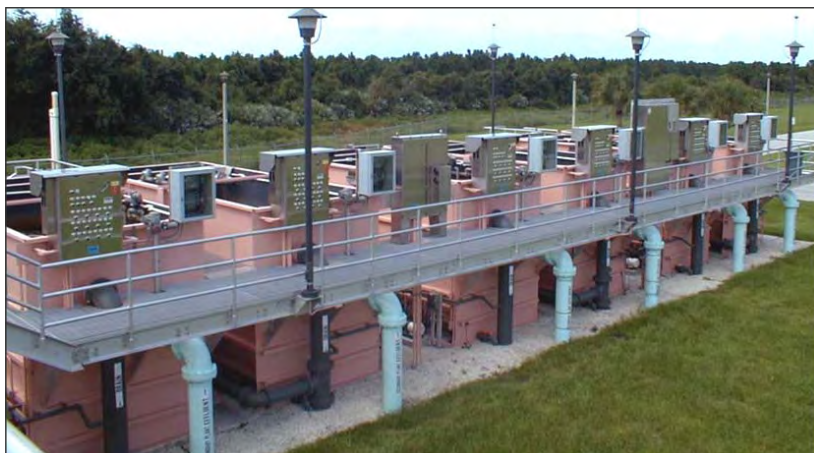
Palm Beach County, FL utilizes (6) 12-disk cloth media filters (30 mgd) for the treatment plant's wastewater reuse program to supply land irrigation.
