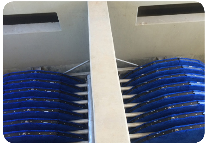
The (2) Aqua MegaDisk ® filters at Talladega, AL are located next to each other in concrete tanks.
