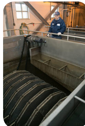
Superintendent, Alan Zerbato visually inspects one of the AquaDisk filter units.
