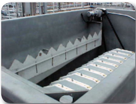
Orange County's North Plant AquaDisk® Filters utilize pile cloth media.
