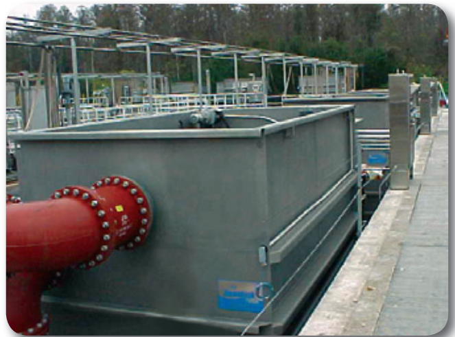
Orange County's North Plant AquaDisk® Filters.
