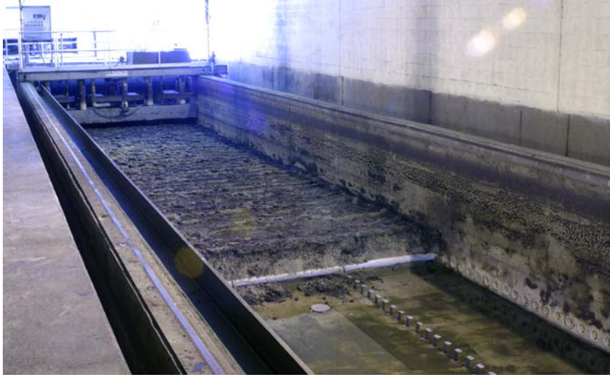
Figure 1: Low Head Shallow Bed Traveling Bridge Sand Filter
