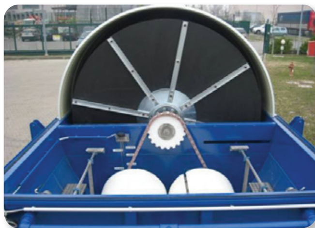
Internal view of the RBC and cloth media drum filters.
